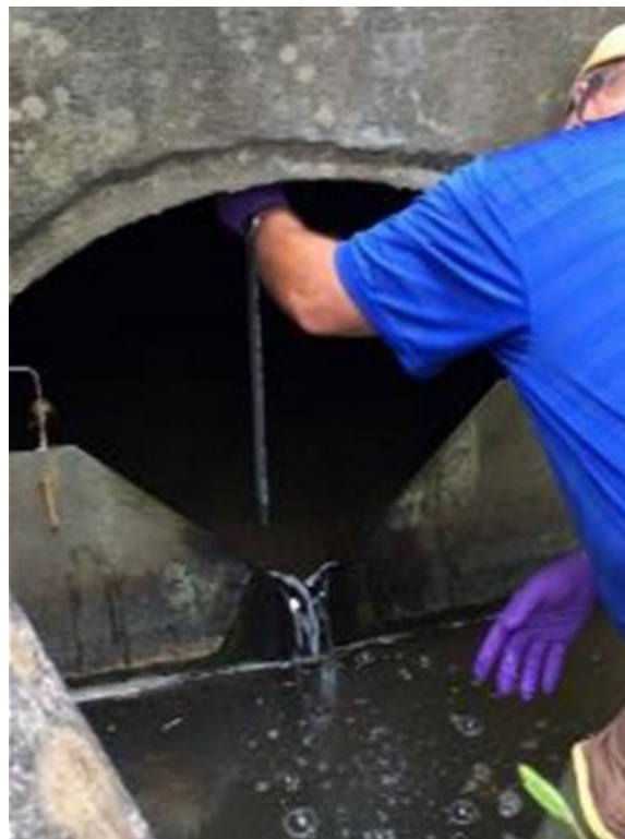
Figure 3.13. Storm water outfall monitoring
